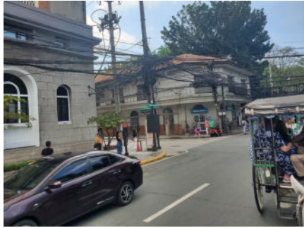
Look at that tangled mass of wires!
